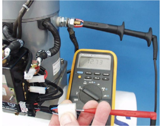
Checking voltage on motor harness to battery negative stud
